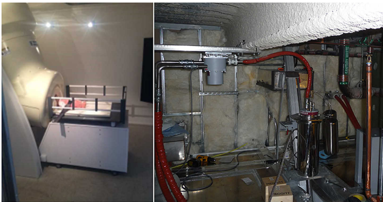
Figure 4. Photos of the closed cycle helium reliquefier installed in a pediatric MEG system at BCH.
